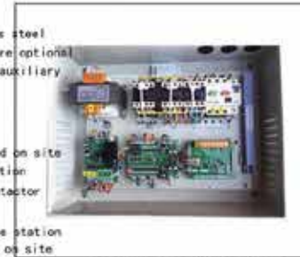
microcomputer control system
